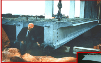
First Bulb-Tee bridge girder pre-tensioned with CFRP tendons, and monitored using Fiber Optic Sensors
